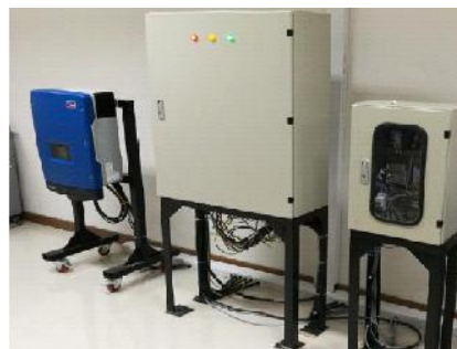
Gambar 3. Inverter on-grid SMA Sunny Tripower TL10000, panel MDB dan panel MTU
