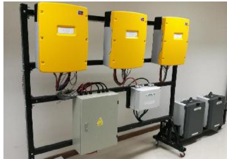
Gambar 4. Hybrid Inverter Sunny Island SI3.0M, Parallel Kit, Fuse Box, dan Li-on Battery 2x5 kWh
