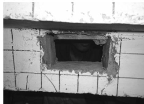
First Crack BLKLB02
