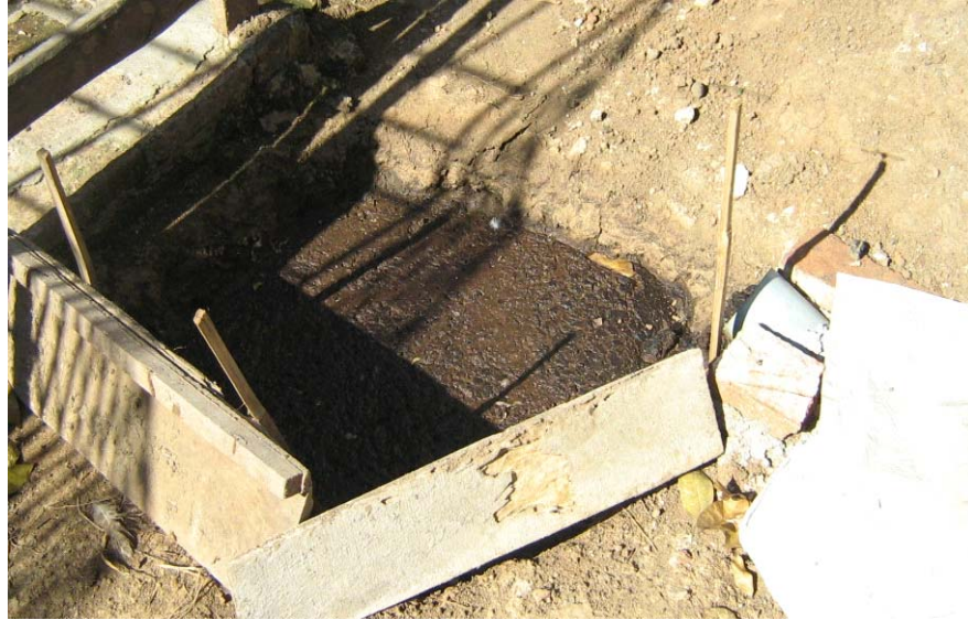
. Gambar 5. Bak Output Digester .
