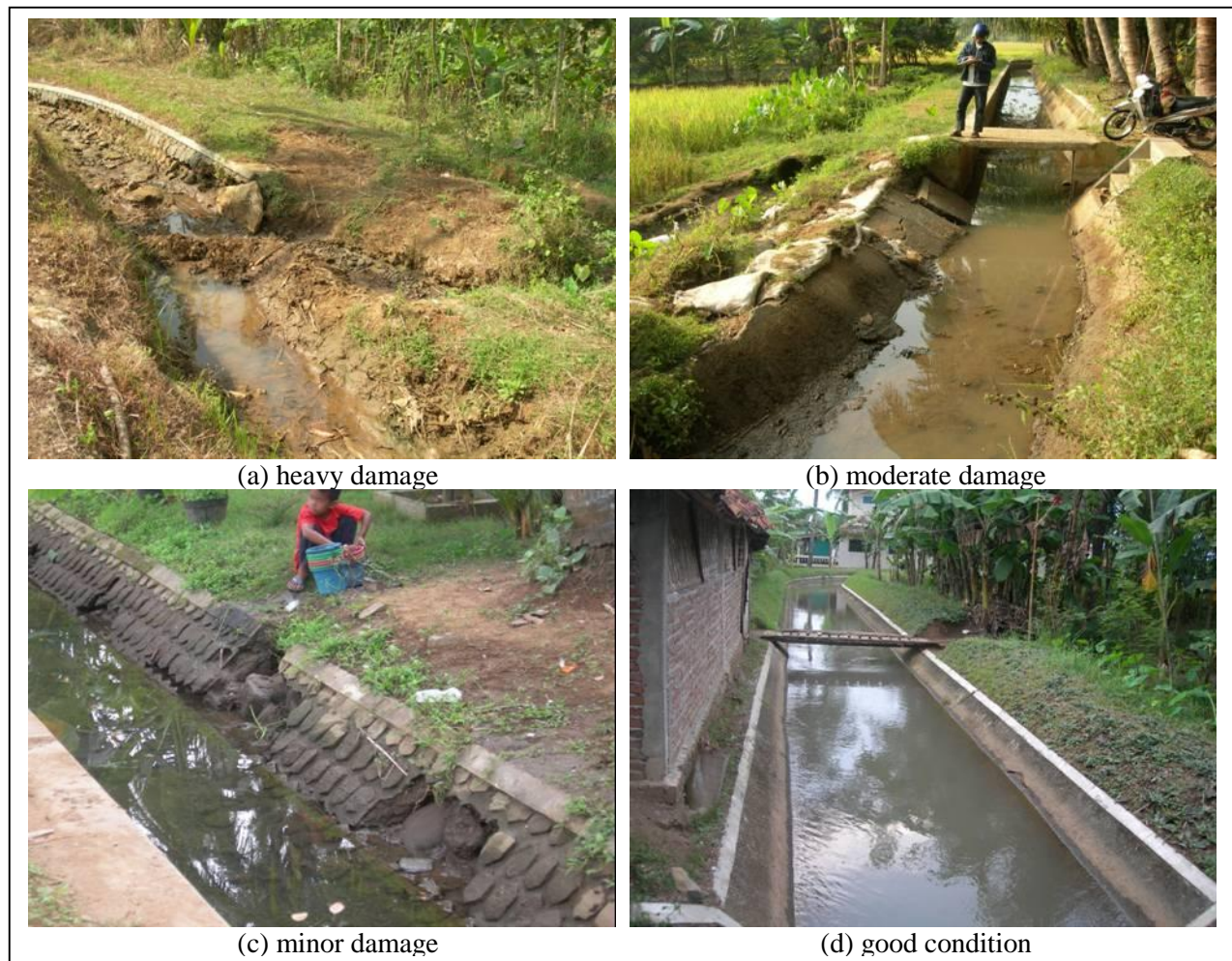
Figure 2. The channel damage condition.
