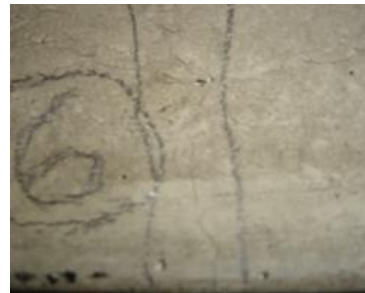
Figure 6. Cracks in the UM beam
