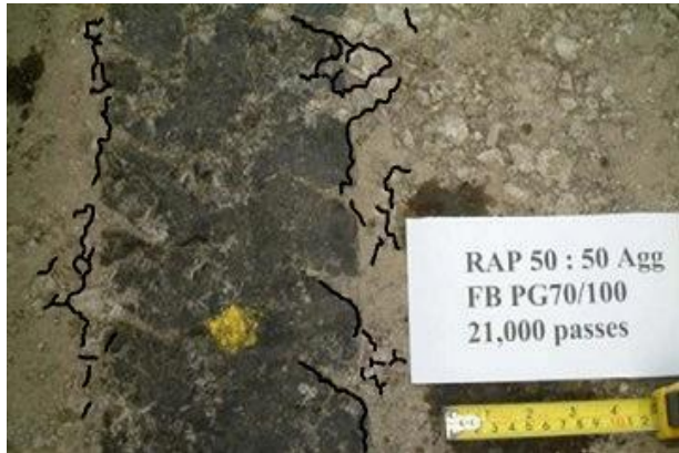
Figure 6. Appearance of longitudinal cracks observed at both sides of the wheel path (coloured black)
