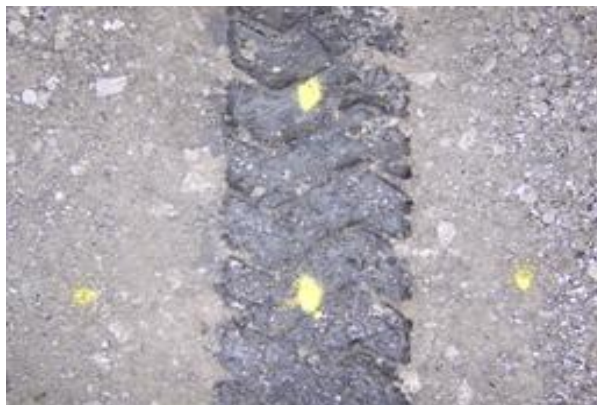
Figure 7. Appearance of the excessive rutting at the wheel path with formation of bleeding
